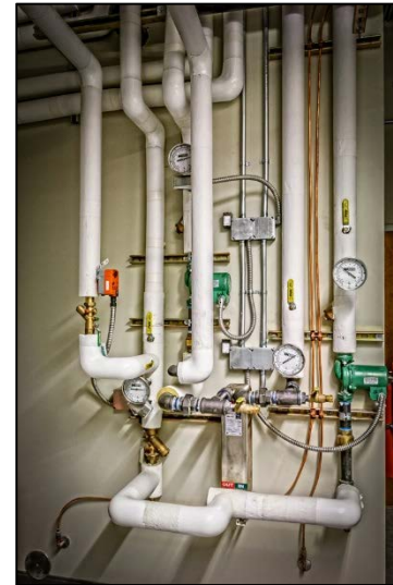
Geothermal Heat Exchanger
