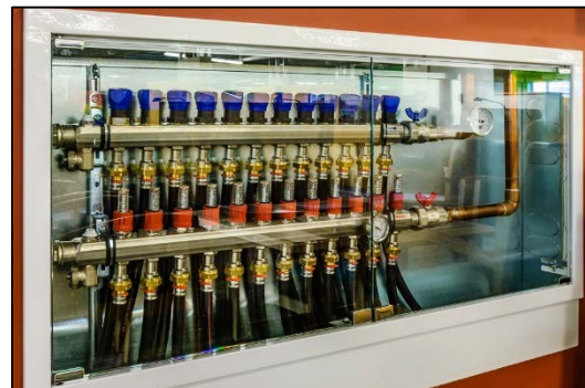
Radiant Slab Manifold Display
